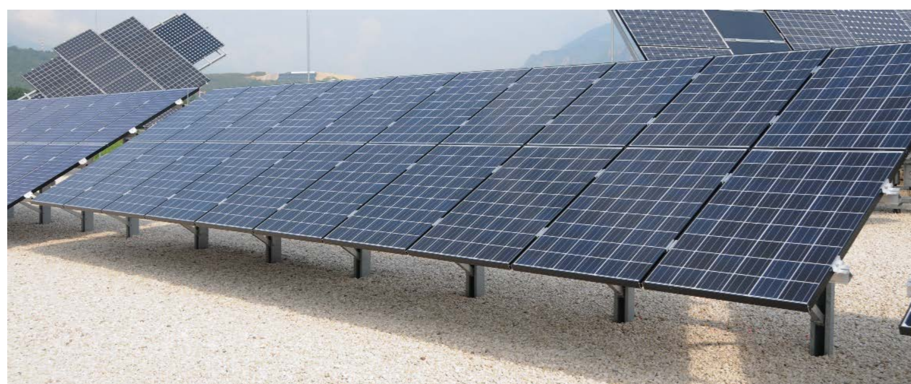
Fig. 1 Studied PV system located in Bolzano (North of Italy).
